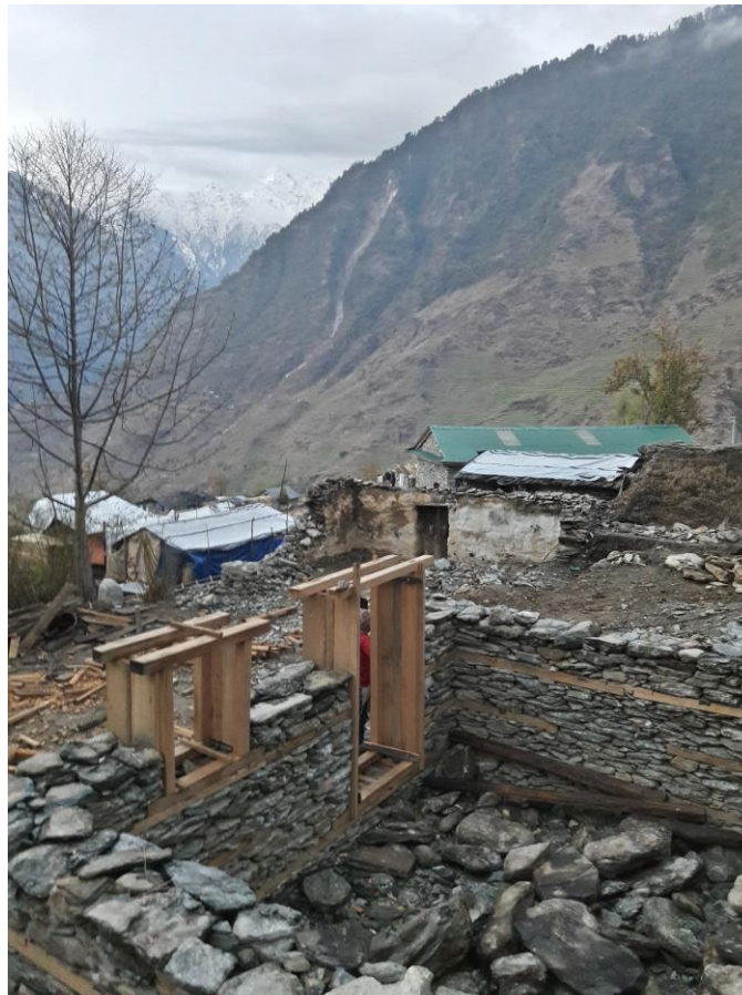
A house under construction in Tipling VDC, Dhading; photo credit National Society of Earthquake Technology-Nepal (NSET).
