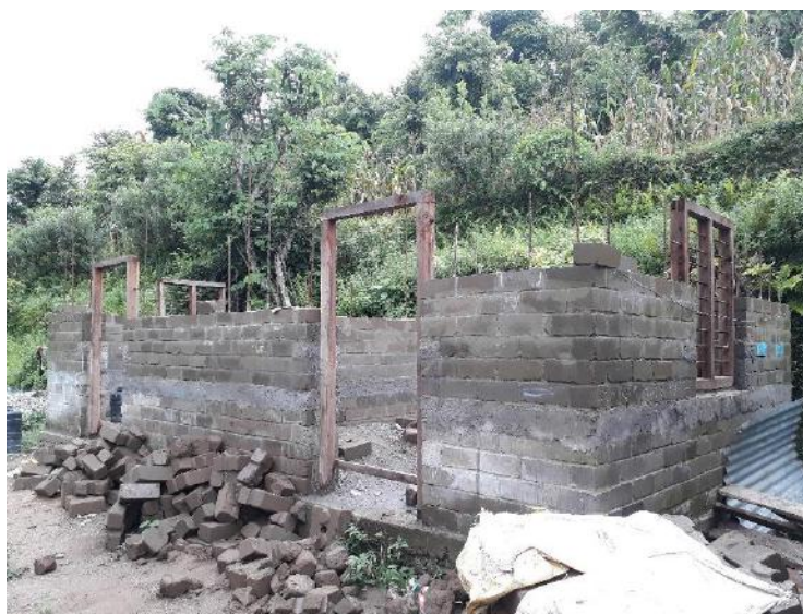
CSEB block demonstration house, Mina Baram, Masel-3, Gorkha, built with support from Build Up Nepal and Save the Children. The CSEB blocks are 60% sand and 30% soil and cost 45-50 NRPs per block.
